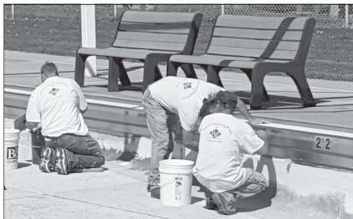
Caulking, crack repairs, and painting should be complete for the start of the summer season.
